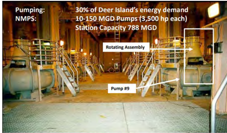
Figure 12: DITP North Main Pump Station - Pump 9
