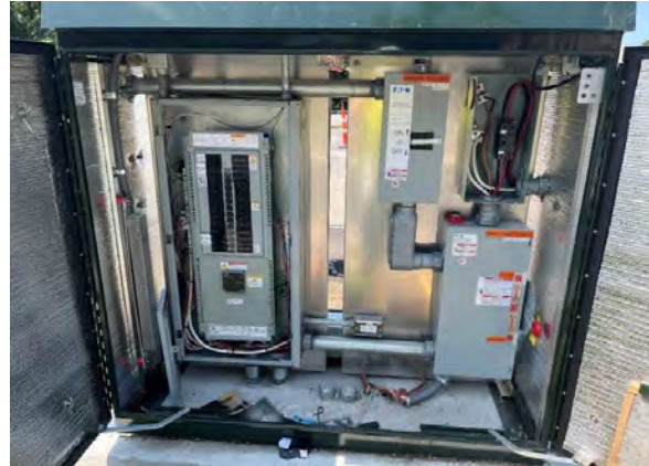
W16 Pedestal Cabinet
